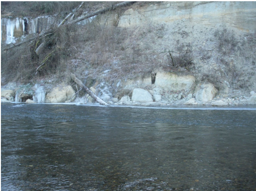
Figure 16. Wedge planer failure of large blocks of sandy material, that is readily reworked by river as part of sediment load. Placing a bankfull bench with J's or Vanes would re-direct flow away from the streambank and allow side slope materials such as shown in Figure 16 to deposit at the base of the slope and on the bankfull bench, such that off-site sedimentation would be greatly reduced.
