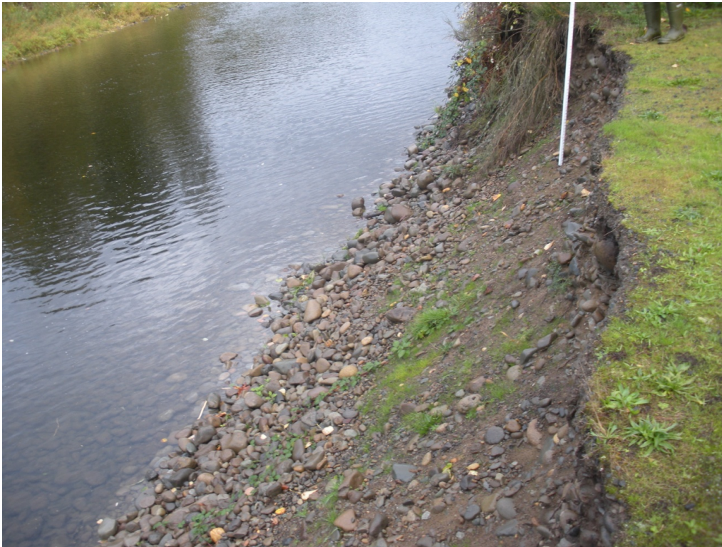
Figure 12 at about RM 9.8 shows a gravel streambank from top to bottom of slope that is failing because fines and sand are being washed out of the gravel and the loss of matrix material causes the streambank to fail. Gravel sloughs and lies at an angle of repose.
