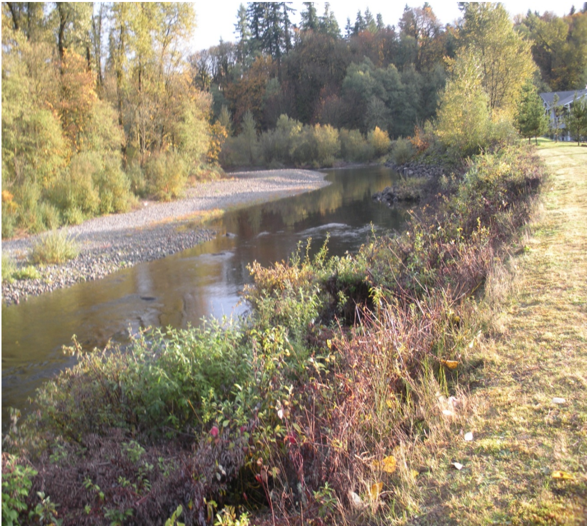
Figure 14 . Rip-rapped section along dike Rm11.6 to 11.7. Brush has been trimmed, but the bank has open areas in rock where one could joint plant or whole plant transplant, if a sufficient moisture regime can be established.
