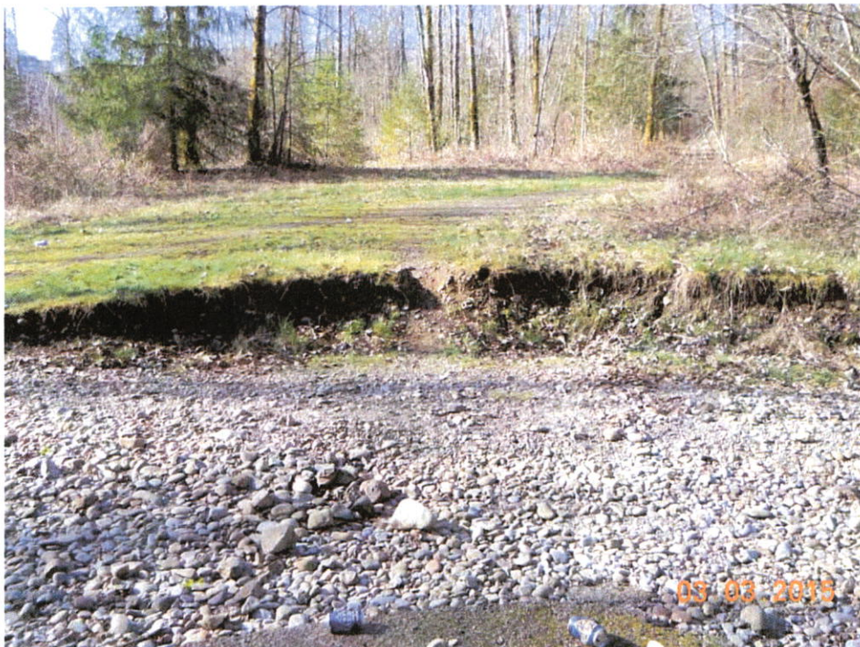
Photo 2. Looking southwest from Location #1 at headcut nick point located at upstream end of secondary floodplain channel.
