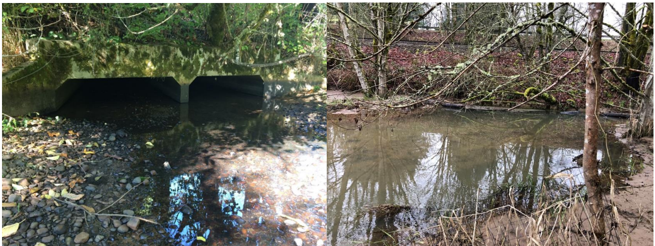
Figure 3– Crabapple Creek, downstream outlet underneath railroad. Photo Orientation: W/looking upstream.
